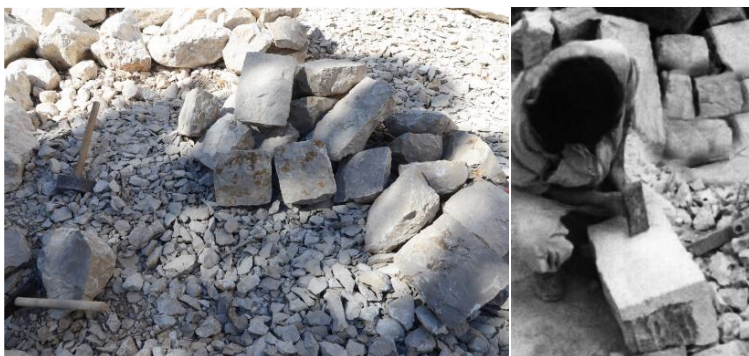
Fig. 23. My pictures: Using old masonry techniques by using old tools; “ Beek ” and “ Shahhouta ”; smoothing the surface of the stone to be used as lintel, in the process of renovating an old house in Achkout built in 1875, now owner Massaad C.
